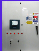
Remote Electrical Enclosure
